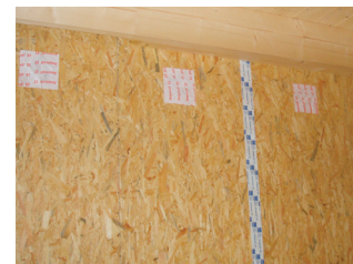
Right: Picture four – Internal view of pre-fab wall panels with joints and insulation holes taped and sealed for air-tightness
